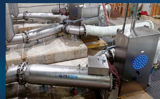
LARGE SCALE AQUACULTURE, USA Large closed vessels for RAS fish farm
