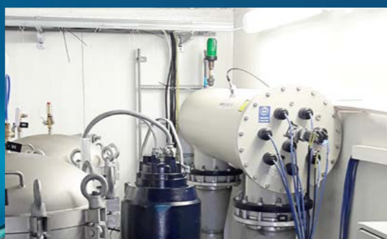
ALLAS SEAS POOL - FINLAND UV system for treating open pool seawater
