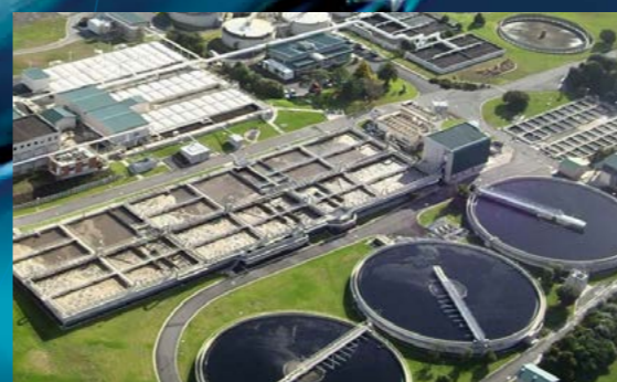
WASTEWATER, CROATIA Channel system for wastewater disinfection
